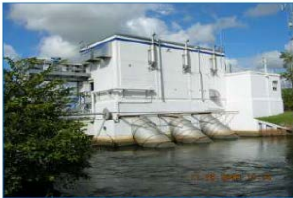
Figure 38 - S-13 Pump station located on C-11 canal at US441 and Orange Drive in Davie, FL. It has a rated capacity of 540 cfs, and can pump approximately 14.5 million gallons per hour (SFWMD, 2007).
