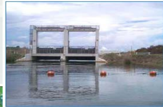
Figure 37 – Typical coastal flood/salinity control structure of the sluice gate type. (SFWMD)
