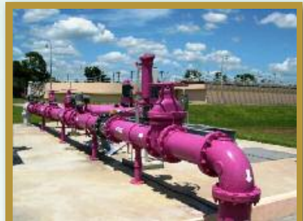
Purple pipes indicate treated wastewater transported for reuse purposes. Photo courtesy of Brown and Caldwell.
